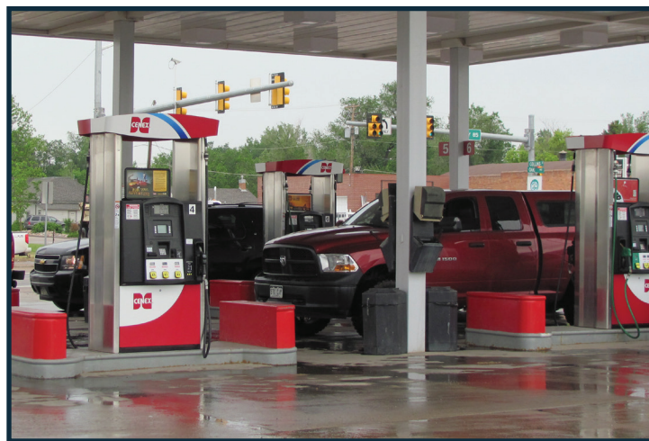
ABOVE: Newly installed Gilbarco Encore® 500 S dispensers.
