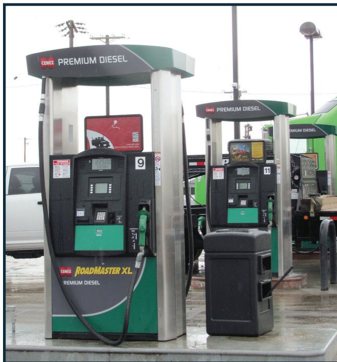
ABOVE: The new Gilbarco Encore® S Ultra-Hi Flow - Masters & Satellite combination dispensers that were added providing additional fueling lanes for Agfinity's customers.
