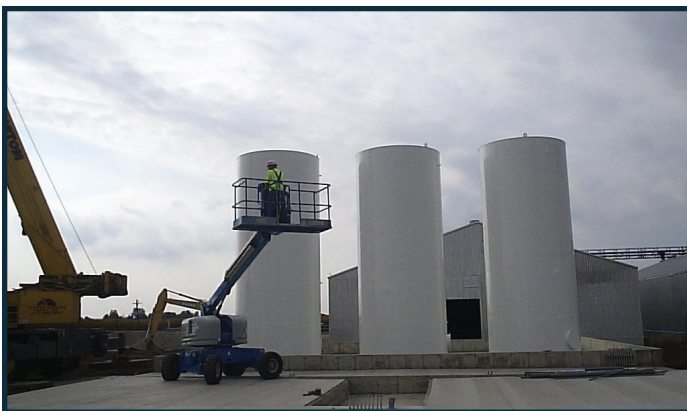
ABOVE: Three (3) 24,000 bulk above ground storage tanks.
